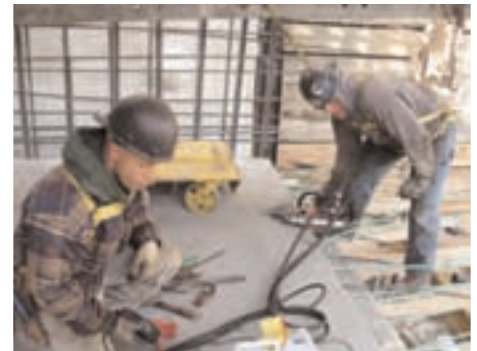
Proper training means these cables are well stressed, but the Local 46 team isn't.
